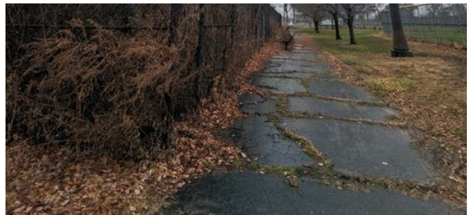
FIGURE 28 Poor Sidewalk Condition.
