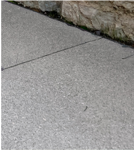
Micro-Etched Concrete Heavy Duty, Sawcut Joints
