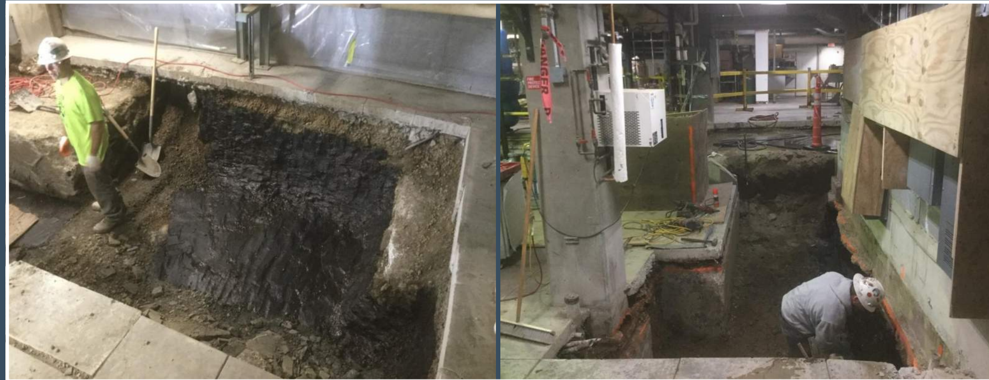
EXCAVATION REQUIRED TO MITIGATE THE CIRCUMSTANCES OF THE EXPANSIVE SHALE FROM EXISTING BASEMENT.
