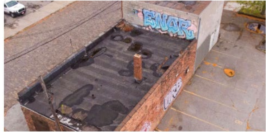
EXTERIOR- ROOF PENETRATIONS AND GRAFITTI
