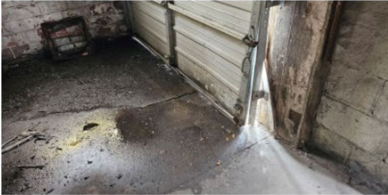
INTERIOR- WATER DAMAGE AND MOLD
