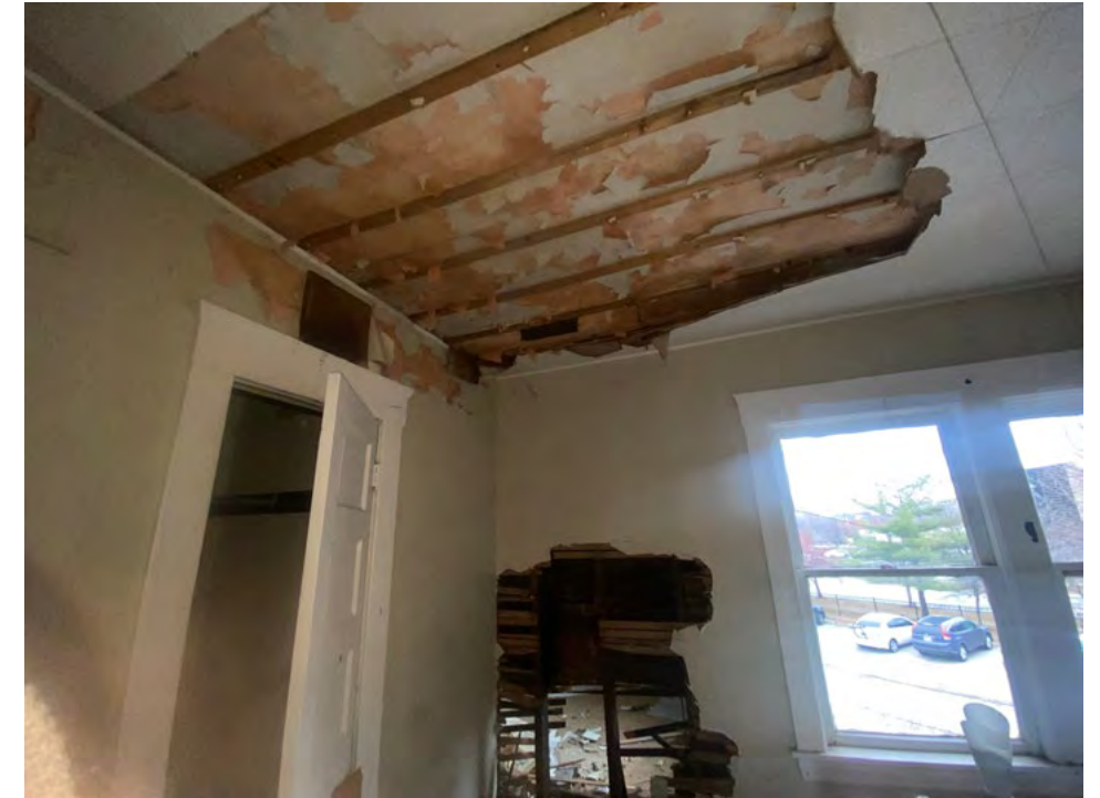
DAMAGED INTERIOR WALLS / CEILINGS
