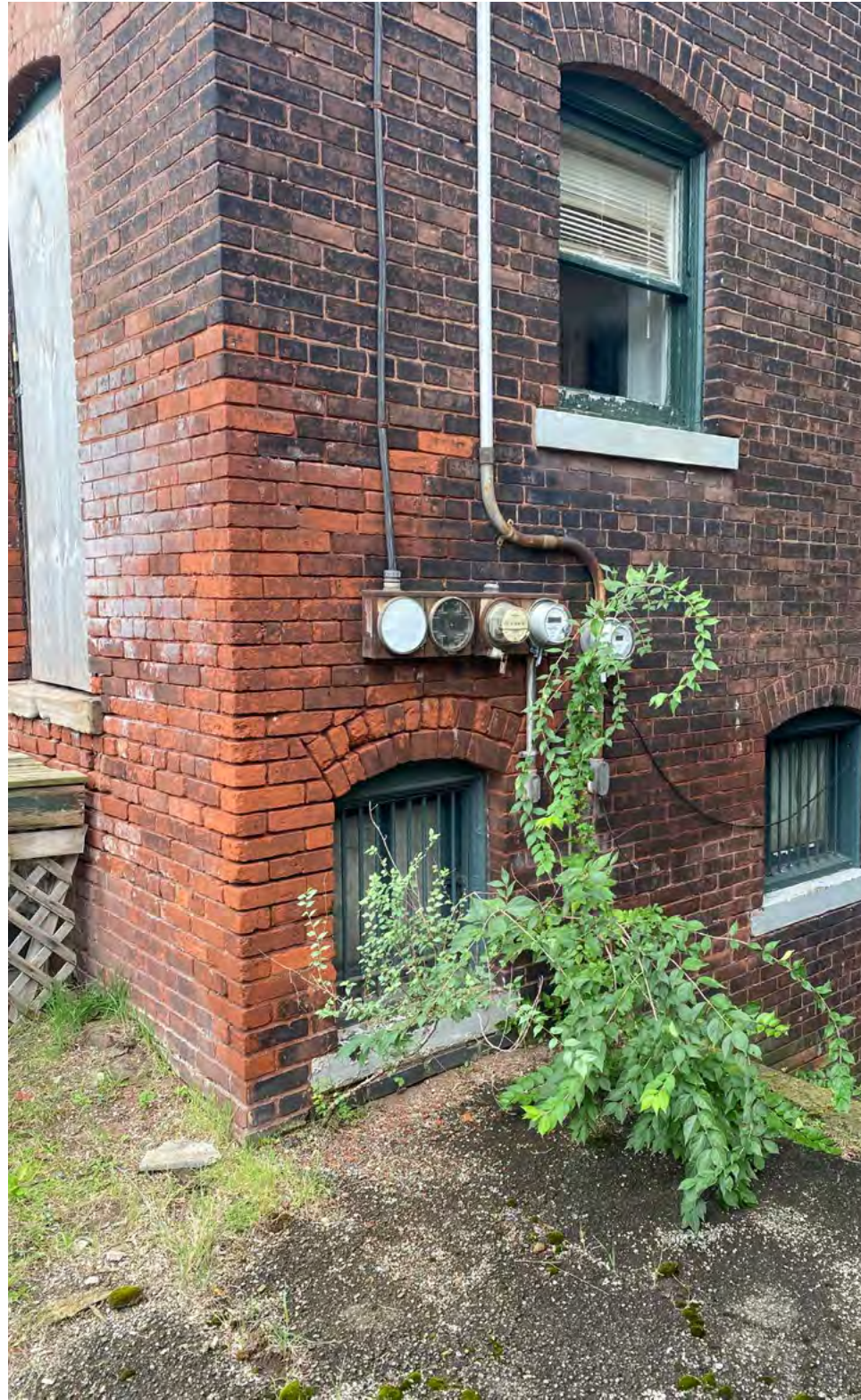
MASONRY TUCKPOINTING / DAMAGED OPENINGS
