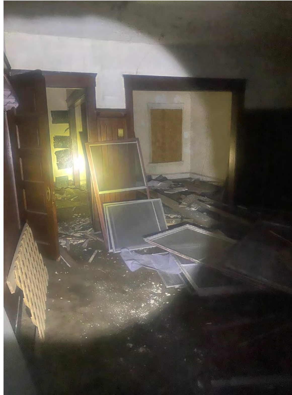
DAMAGED INTERIOR / FAILING WINDOW OPENINGS
