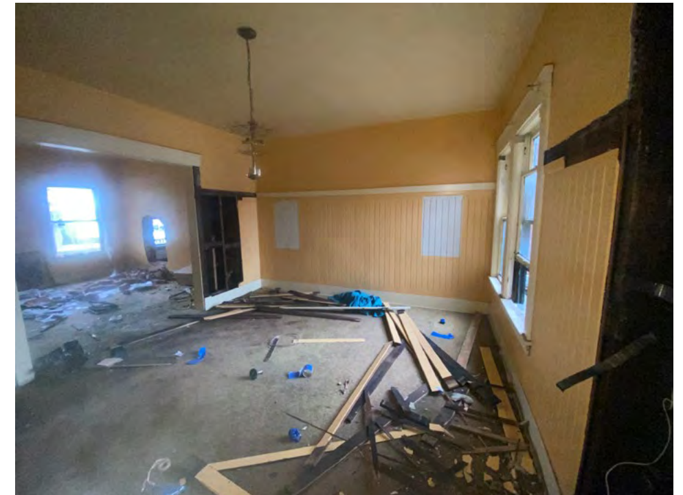
DAMAGED INTERIOR WALLS / CEILINGS
