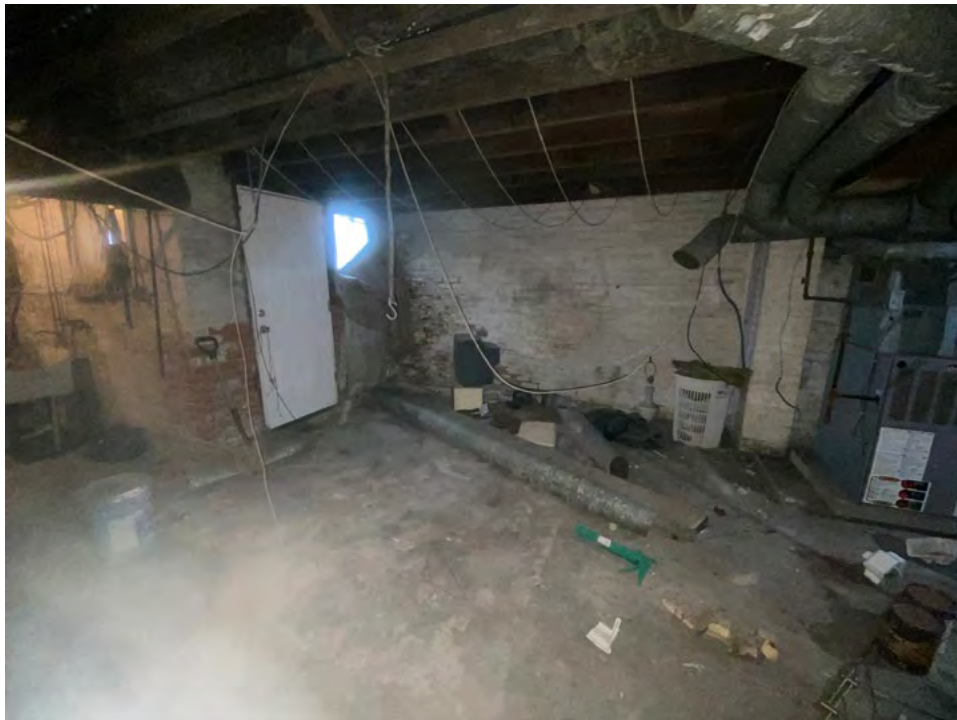
DAMAGED PIPES / LEAKAGE FROM BROKEN WALLS
