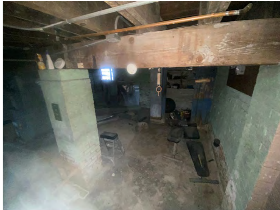
DAMAGED PIPES AND MECHANICAL SYSTEM
