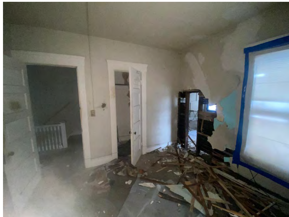
DAMAGED INTERIOR / FAILING WINDOW OPENINGS
