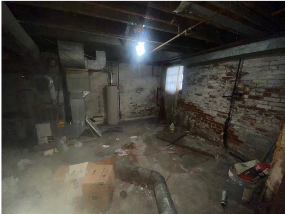
DAMAGED PIPES / LEAKAGE FROM BROKEN WALLS
