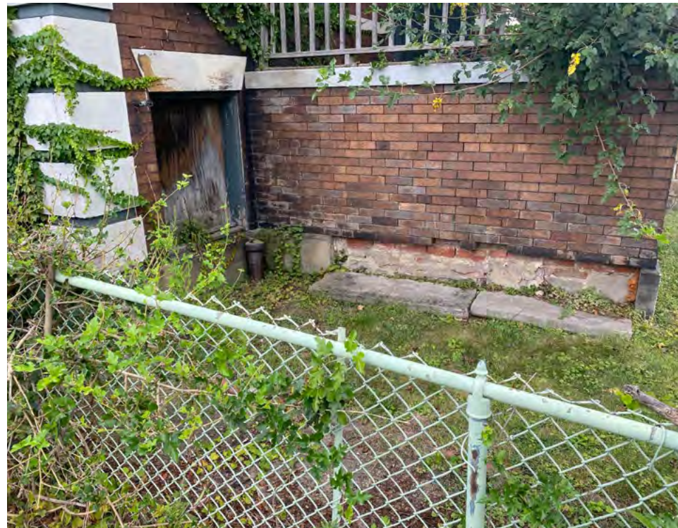
MASONRY TUCKPOINTING / DAMAGED OPENING
