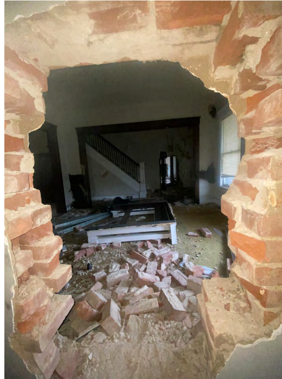
DAMAGED INTERIOR / BROKEN WALLS
