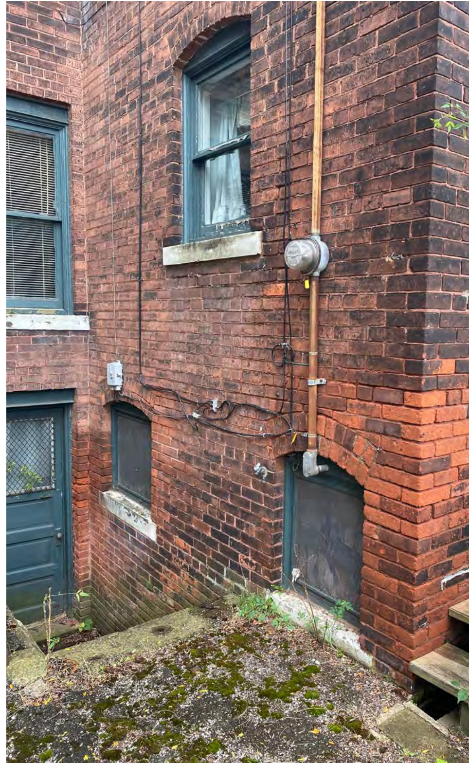
MASONRY TUCKPOINTING / DAMAGED OPENINGS
