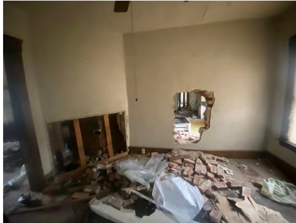
DAMAGED INTERIOR / BROKEN WALLS
