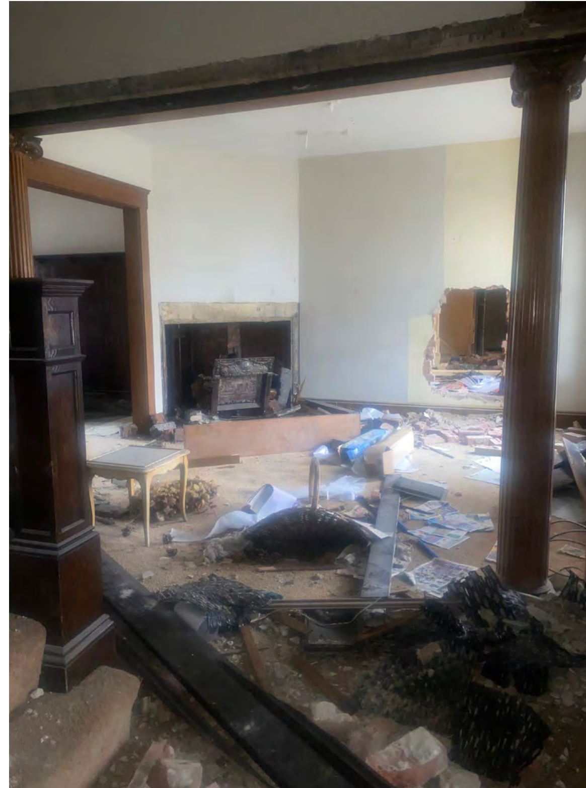
DAMAGED INTERIOR / BROKEN WALLS
