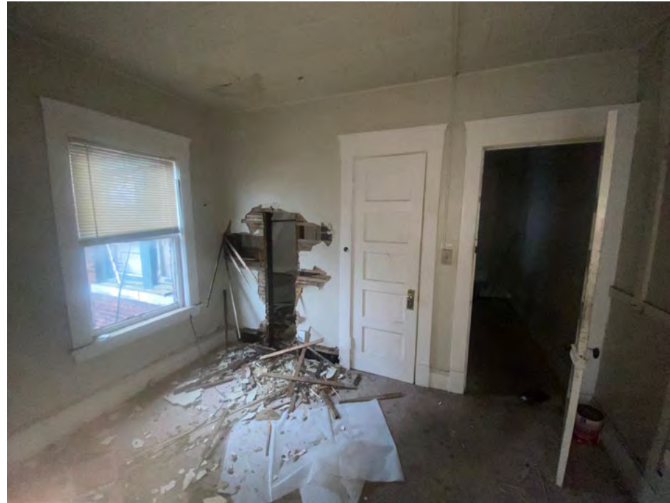
DAMAGED INTERIOR / BROKEN WALLS
