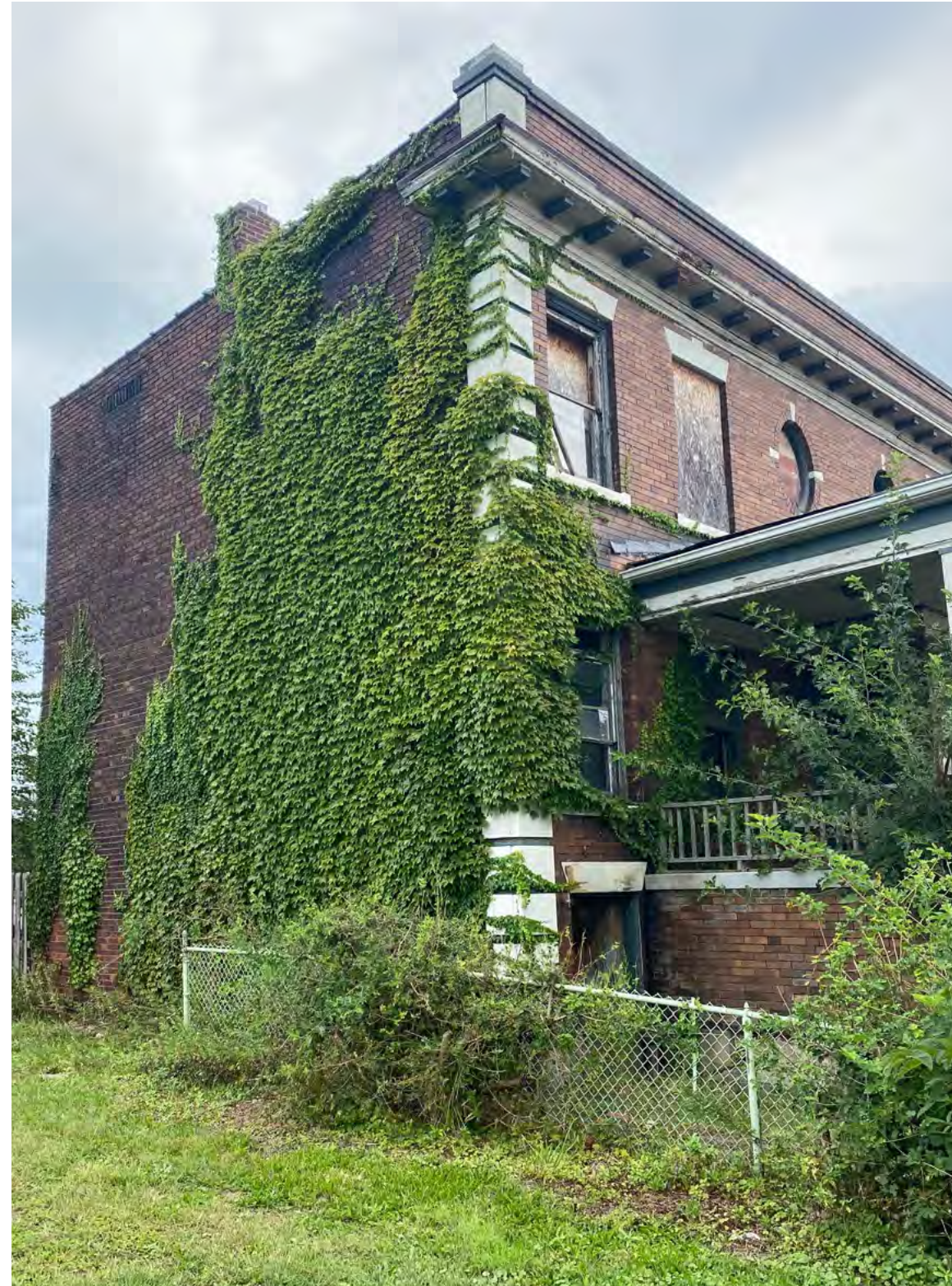
MASONRY TUCKPOINTING / DAMAGED OPENINGS
