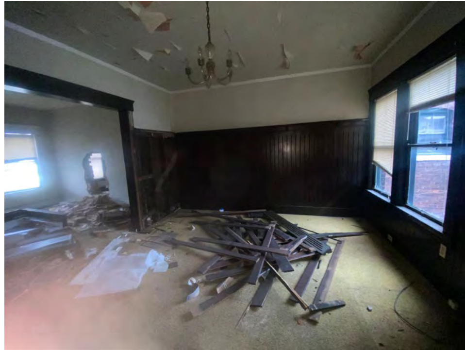
DAMAGED INTERIOR WALLS / CEILINGS
