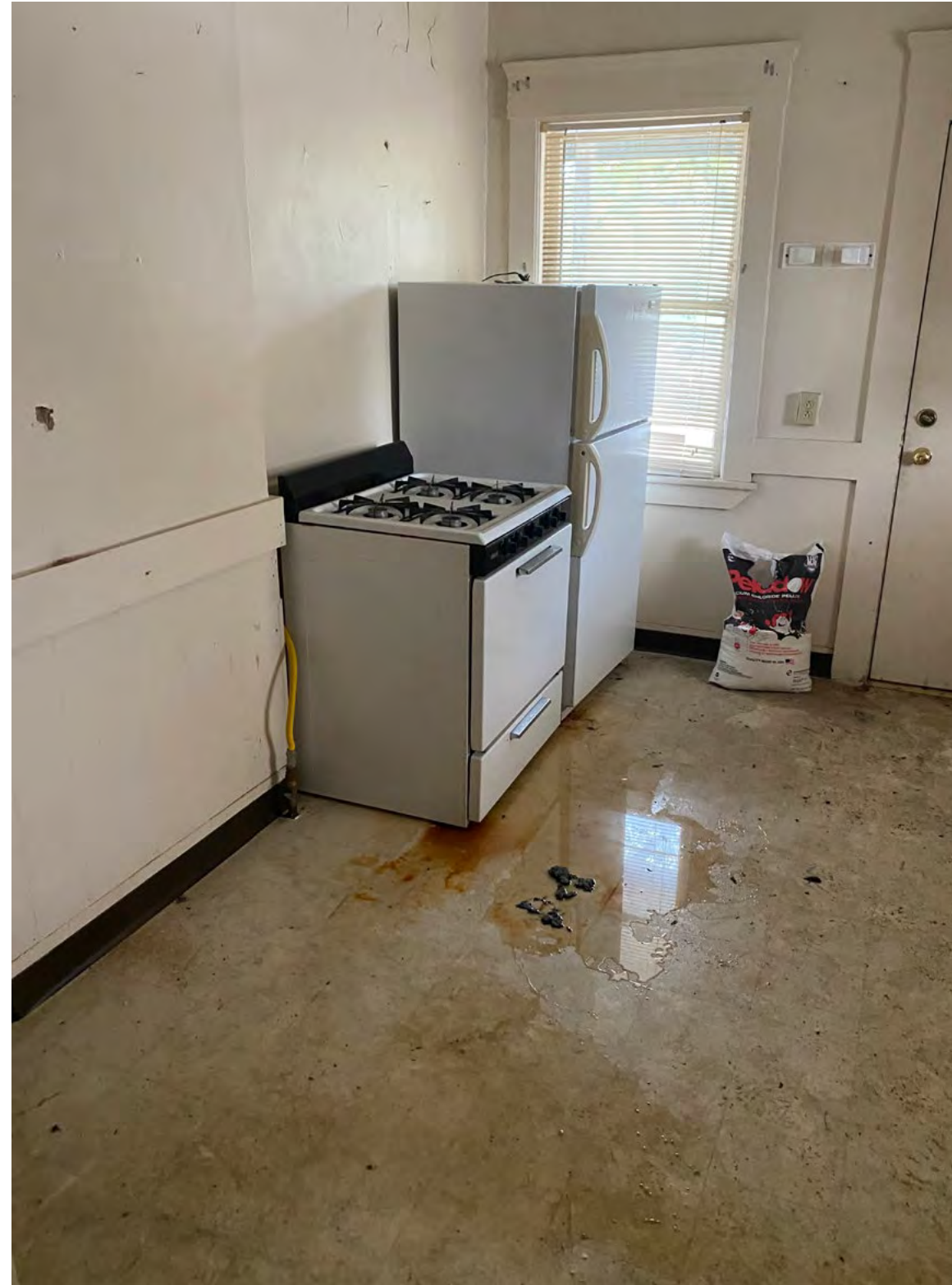
DAMAGED INTERIOR / LEAKAGE
