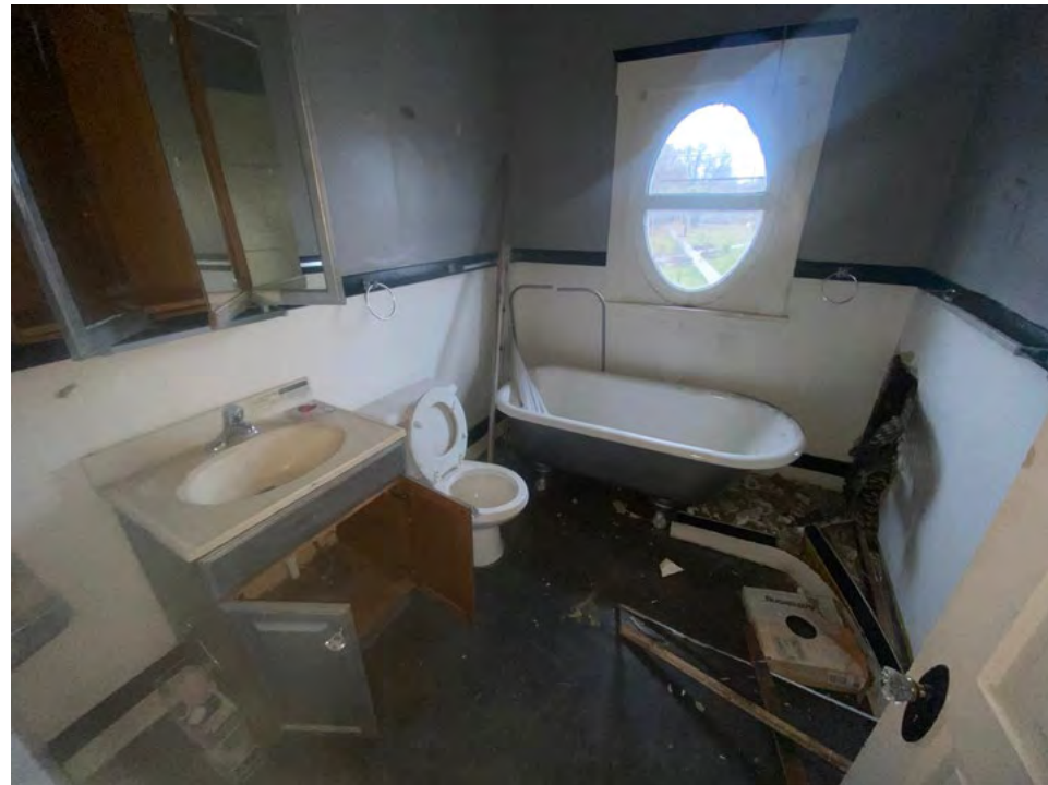
DAMAGED PLUMBING AND MECHANICAL SYSTEMS
