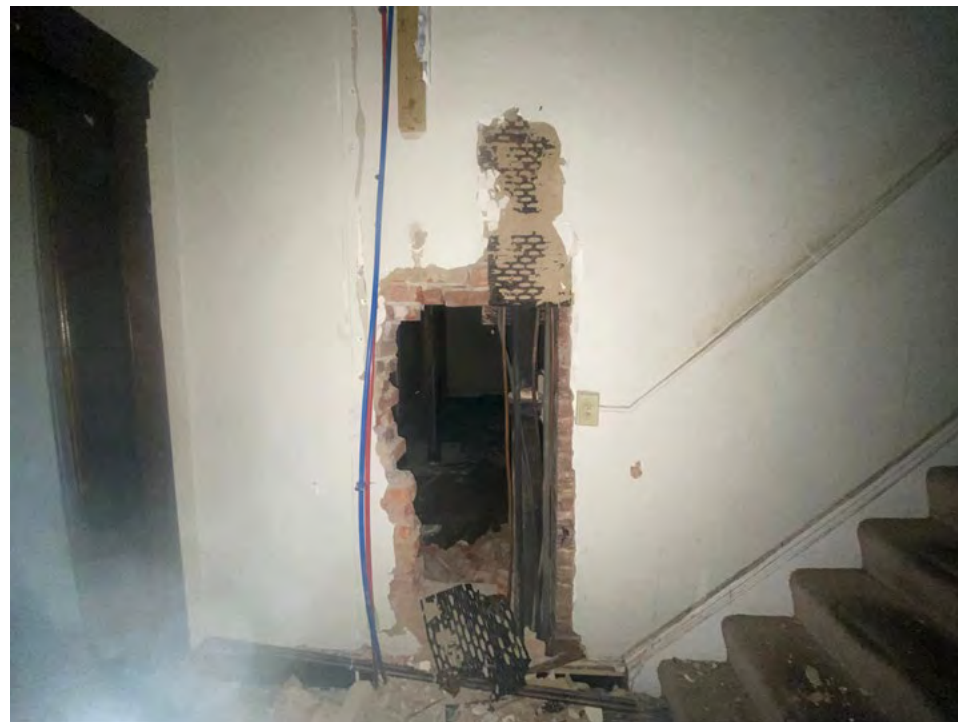
DAMAGED INTERIOR / BROKEN WALLS
